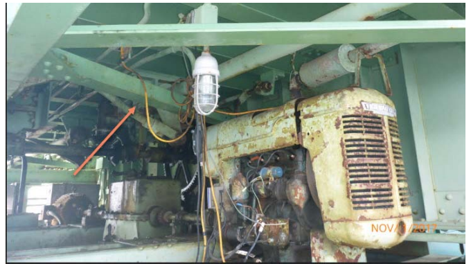
Aging Generator at Gwynn's Island Bridge
